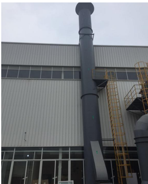
18mDA001 熔铸废气排气筒
